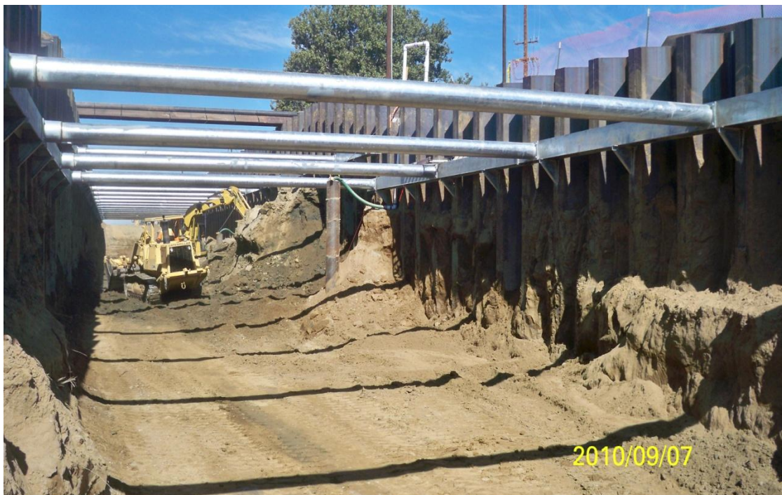
West Bay Subcontractor Meyer excavating in the canal structure to concrete sub grade elevation.
