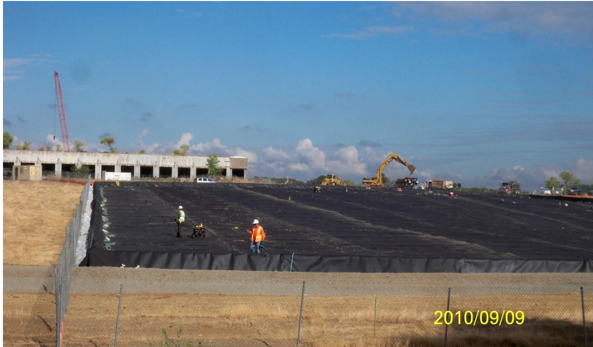
West Bay Subcontractor Sierra Geosynthetic Service installing the geomembrane to stockpile landfill excavation material.
