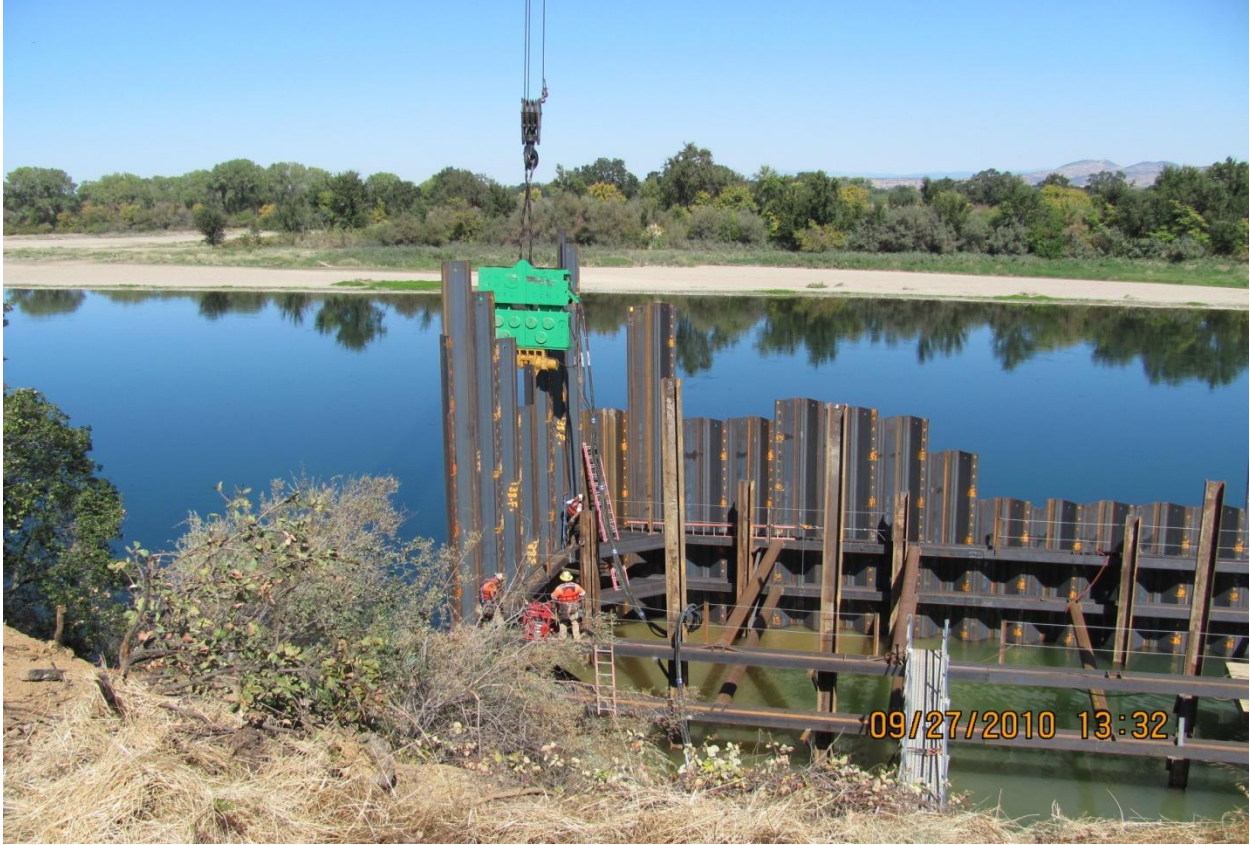
Balfour Beatty working on Red Bluff Pumping Plant & Fish Screen Cofferdam Sheet Pile Driving.
