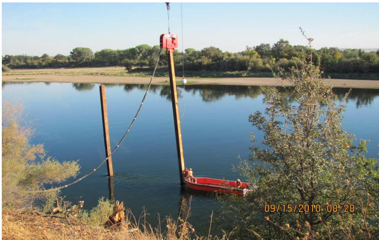
Balfour Beatty employees driving sheet piles for upstream end of fish screen cofferdam, sheet pile guides.
