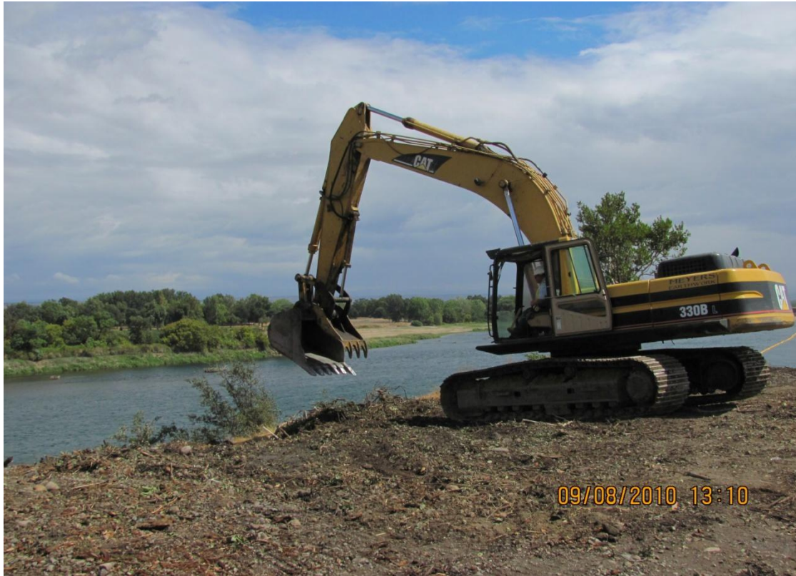
Balfour Beatty Subcontractor Meyer's tracked excavator working on clearing & grubbing in the area of the future fish screen.
