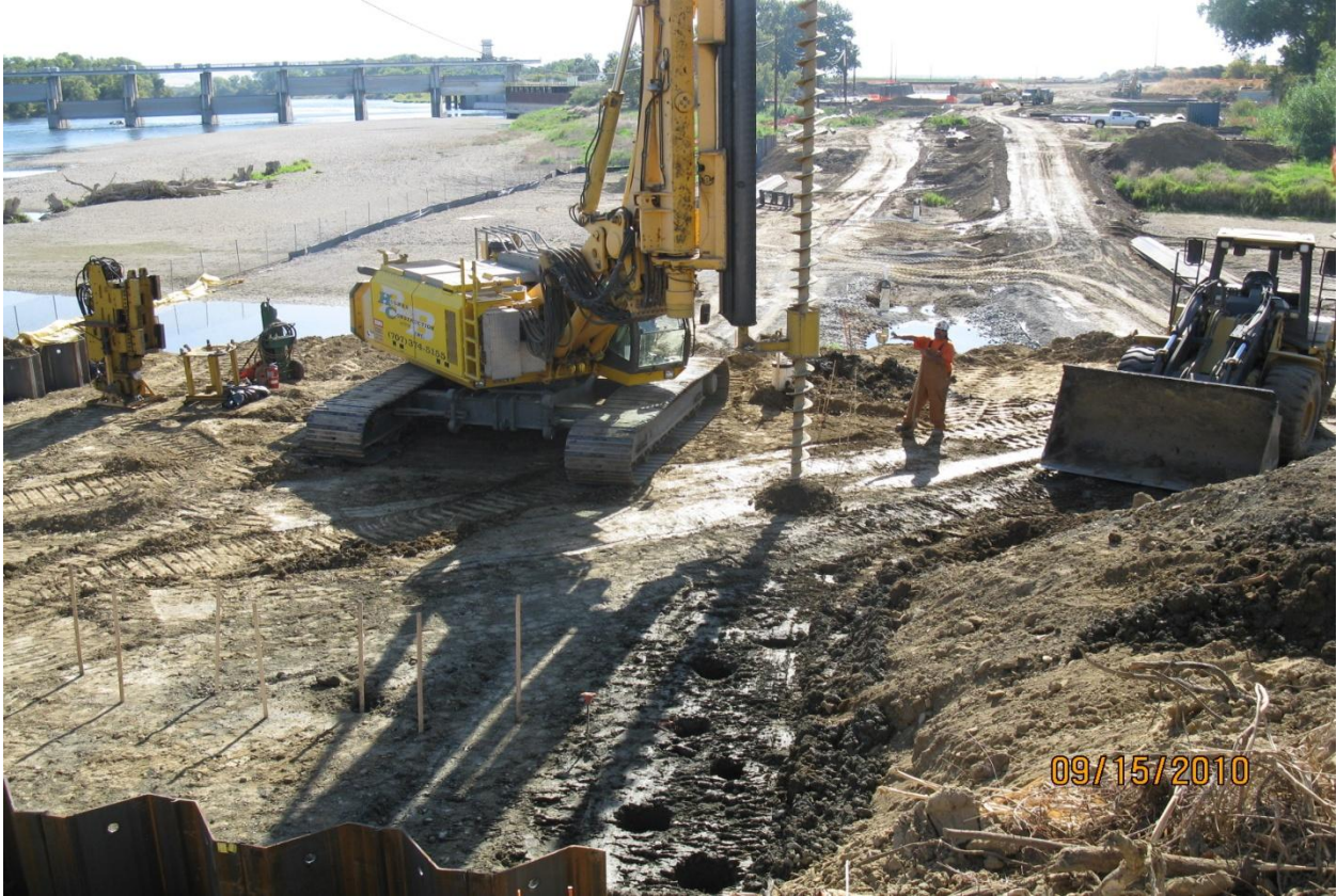
West Bay Builders Subcontractor Hughes Construction pre drilling before installing sheet piles.
